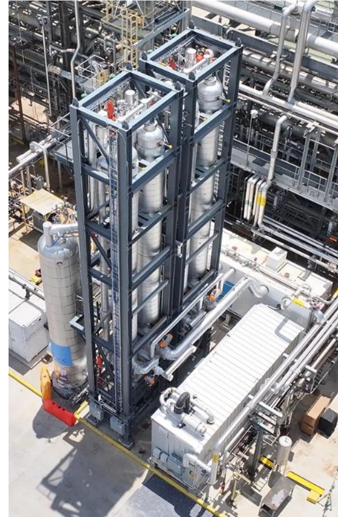
Carbon America's FrostCC™ deployed at NCCC
