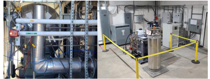
Figure 10: SOFC pressure vessel and BOP in test cell (left), SOFC/GT supporting equipment (right)
