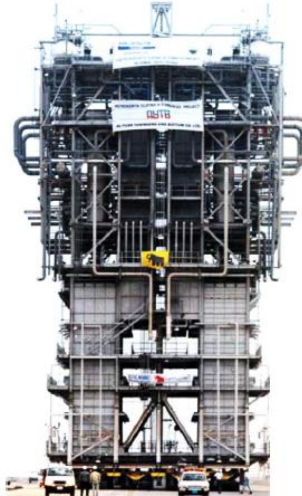
Steam Cracker Furnace (600 tpd ethylene)
